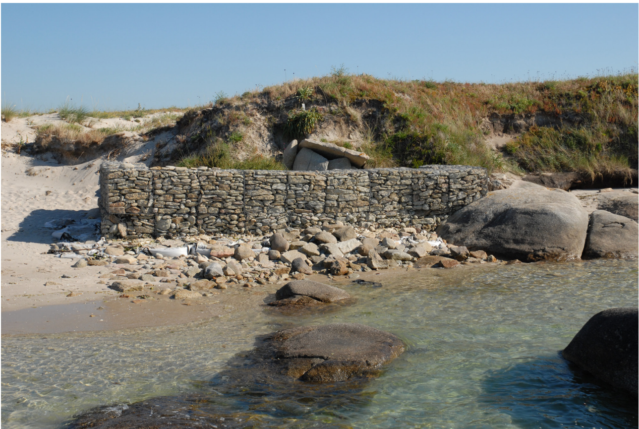
Fig. 6 – Dry-wall protection for monument M4 in Guidoiro Areoso (built in 2011; 17/06/2014).
